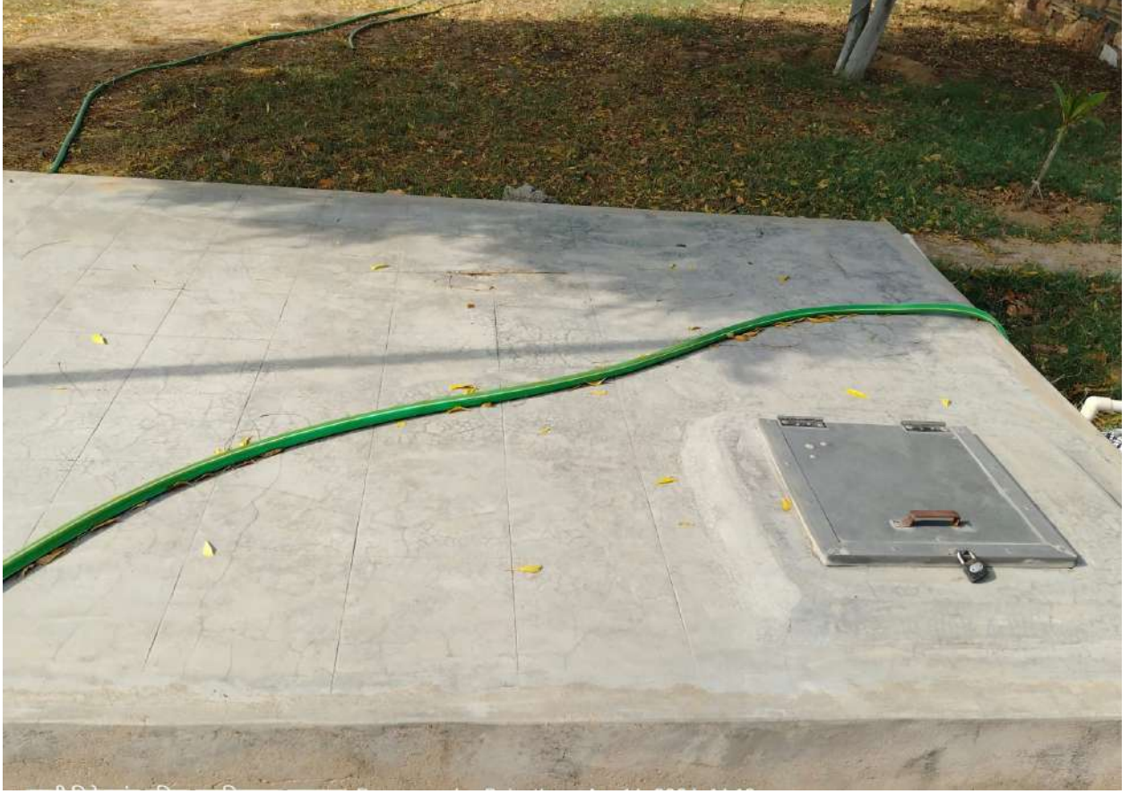
UG WATER TANK
