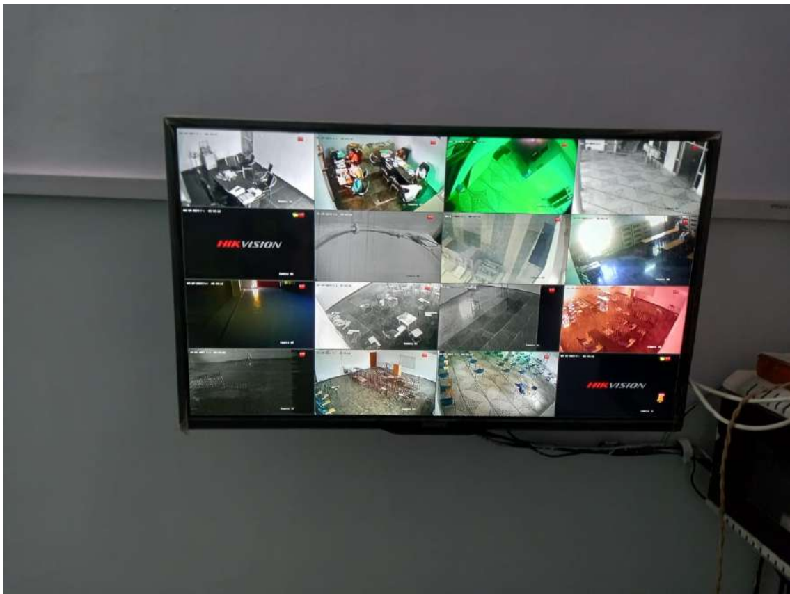
CCTV Surveillance of All Cameras through Principal Office
